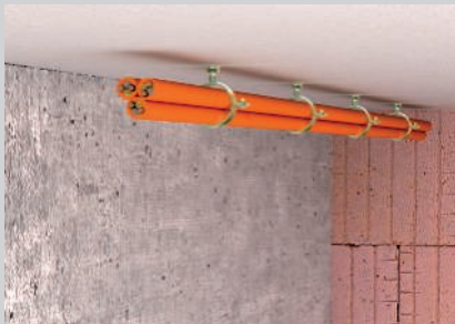
Bundled cable routing under the ceiling.
