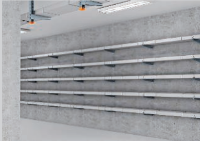
Cable tunnel with bandages in power stations.
