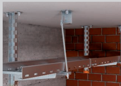
Attachment of the threaded rod in the fire protection clamp.
