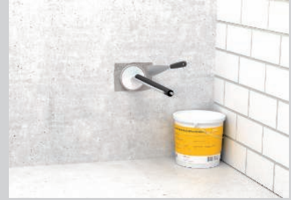
Adjust the foam plugs to installations using a knife and create smoke gas-tight sealing of the sealings using the ASX coating compound.
