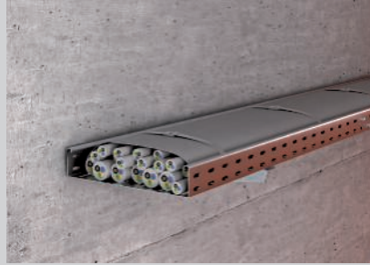
Complete encasement of the cables in a cable run as wall mounting.
